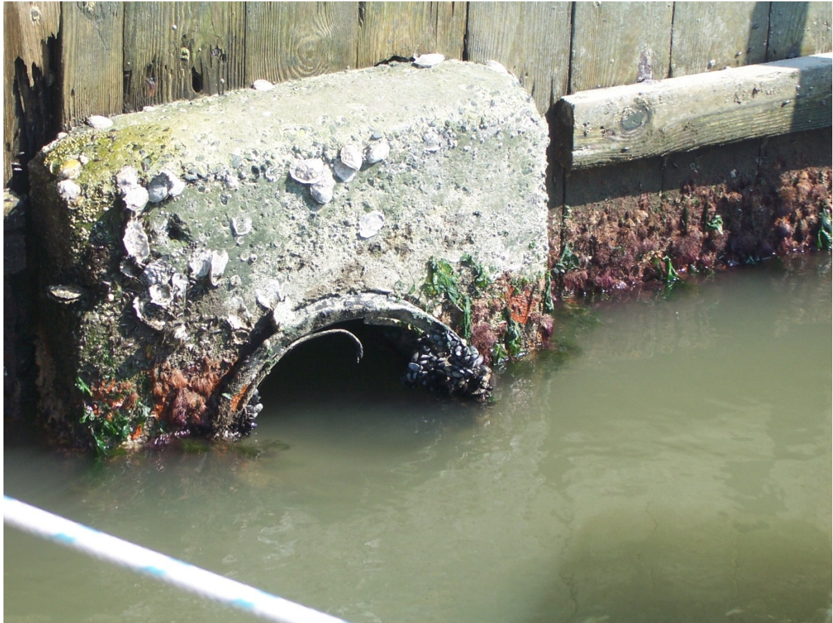
Corrugated metal storm drain pipe with tidal influx
