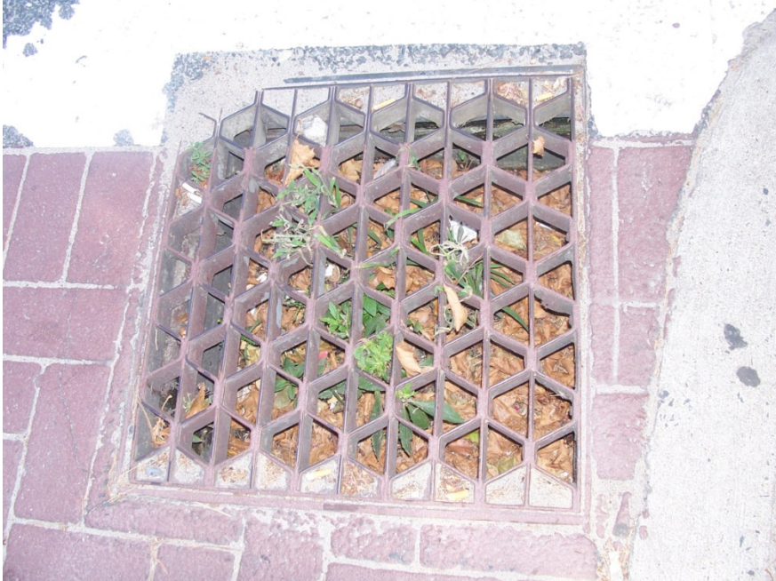
Storm drain in need of clean-out due to leaf debris
