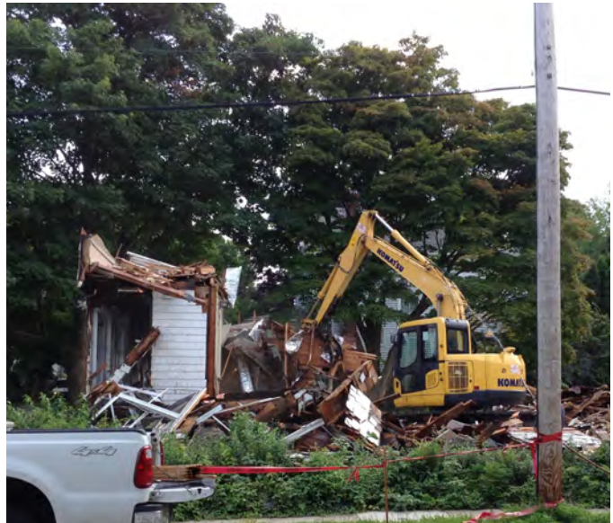
Figure 7. Regulations are but one tool to avoid the outcome of demolition. (Photo by author.)
