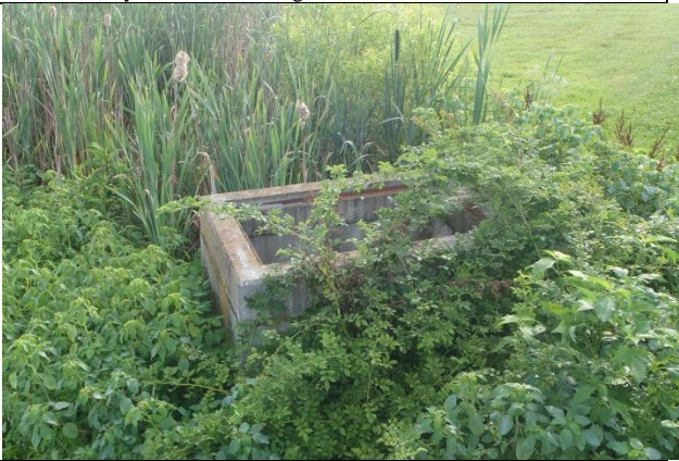
17E Control structure with grate missing
