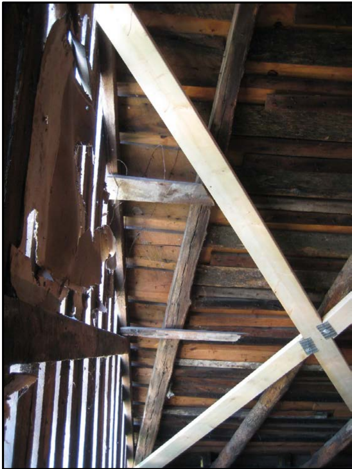
Figure 7. Slave quarter interior east side of roof (2015); original end rafter has shifted @2' to the south; boards of irregular width were installed to span the gap between the original end rafter and the 20C replacement.
