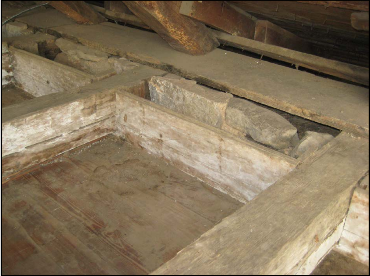
Figure 22. Slave quarter attic detail (2017); horizontal siding boards for room 504 extended to the underside of the original attic floorboards; the underside of the floorboards and the exposed joists, as well as the siding boards, were whitewashed.
