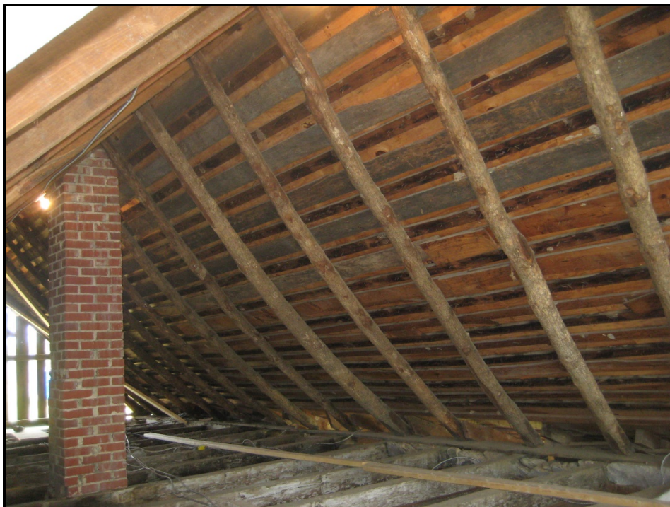
Figure 4. The original pole rafters on the east side of the slave quarter roof shifted between 2' and 2'6" to the south (2015); the existing brick chimney is a 20C replacement of the original.
