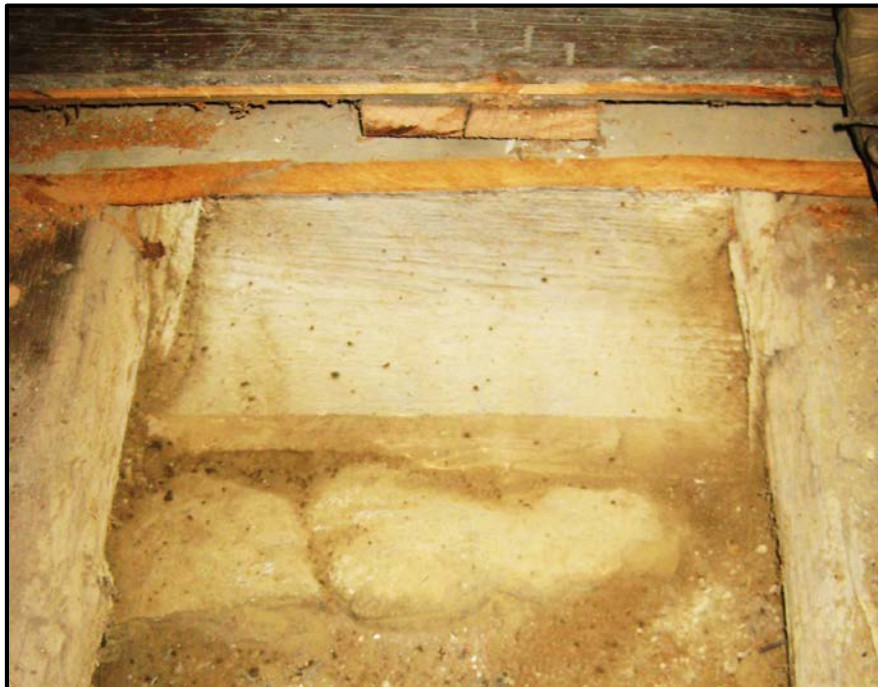
Figure 19. Slave quarter NW corner, interior (2015); joists notched over flat sill, two levels of flooring separated by nailers/spacers for second floor (room 507).
