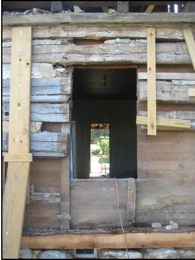
Figure 14. Slave quarter SW window opening (2015); stud and siding boards installed ca. 1917 in room 504 cut to widen opening.
