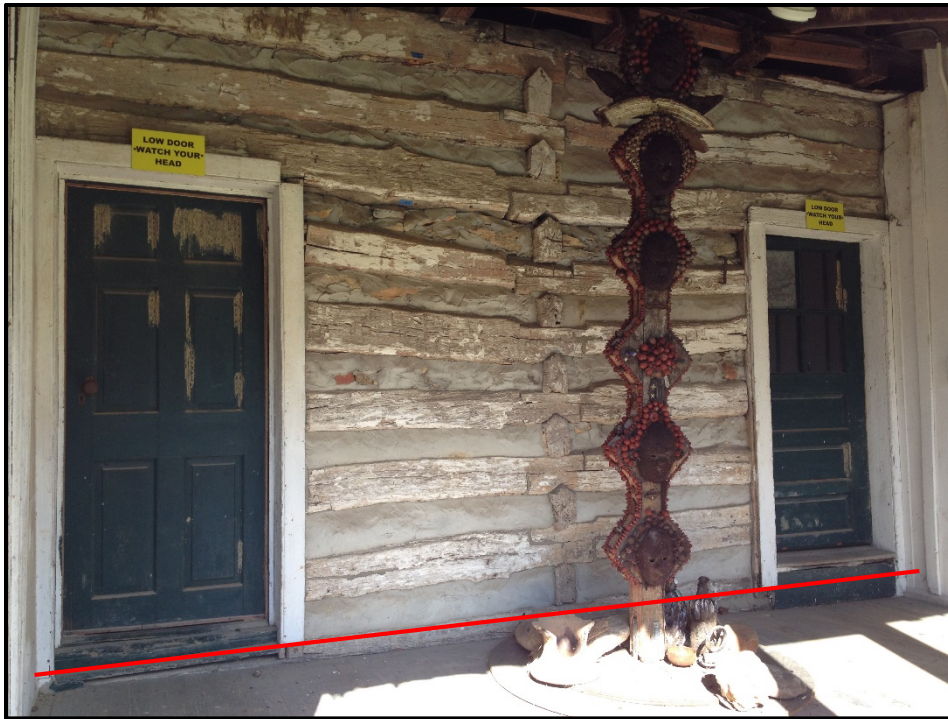
Figure 16. Slave quarter east façade (2015), two original exterior doorways; architraves for both doorways likely installed ca. 1861, cut evenly to suggest earlier floor level of porch (red line).
