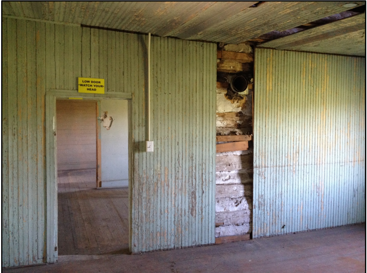
Figure 20. Slave quarter, interior view (2013); south wall room 506, vertical beaded planks applied to log walls and ceiling, hole and thimble for stove pipe visible in portion of exposed logs; plaster board applied to south wall of room 505; horizontal plank siding on south wall of room 504.
