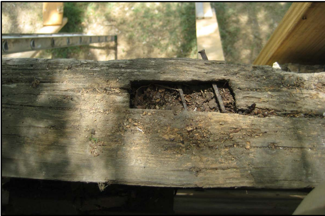
Figure 9. Slave quarter south gable, open stud mortise with cut nails (2015).
