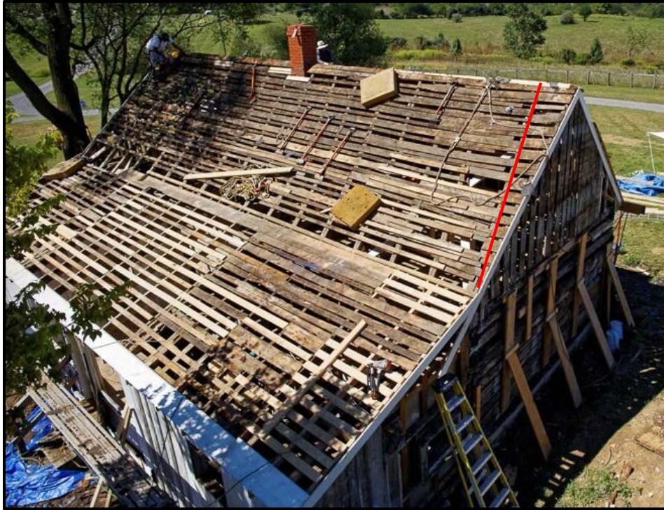
Figure 3. The Clermont slave quarter east side roof frame after shingles and plywood deck was removed (2015); note the severe southward lean of the main roof rafters.
