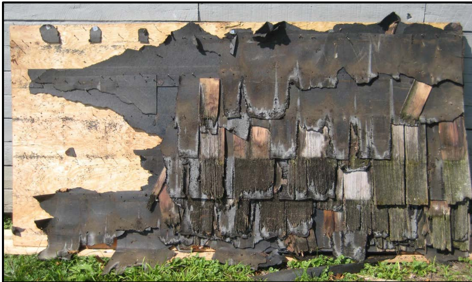
Figure 24. Remnant of 1970 cedar shingle roof, underlain by tarpaper and attached to plywood decking (2015).
