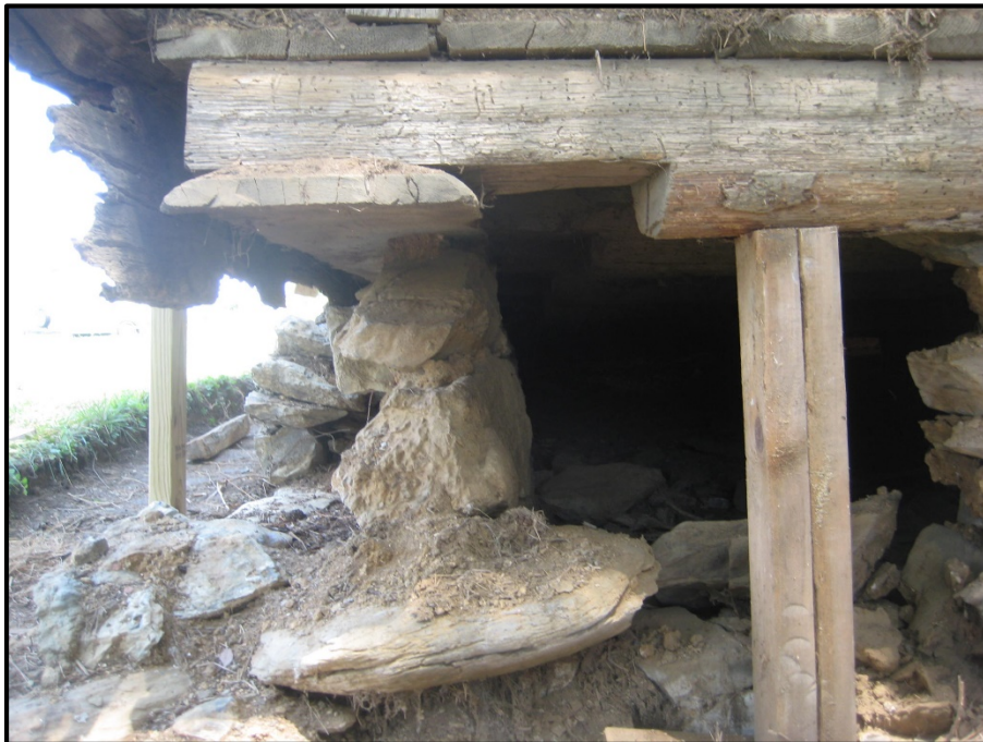
Figure 18. Slave quarter SW corner (2015); end joist notched to lap over flat sill resting on interior portion of foundation.
