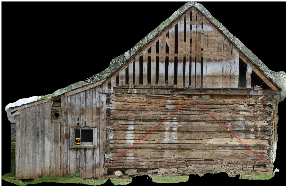
Figure 10. North gable after horizontal siding removed from both the gable and log wall, and after vertical siding removed from the log wall (2015). The ghost of wood brace in the form of an inverted V is visible on the log wall; the deteriorated mortises are visible at the c of the gable end girt.
