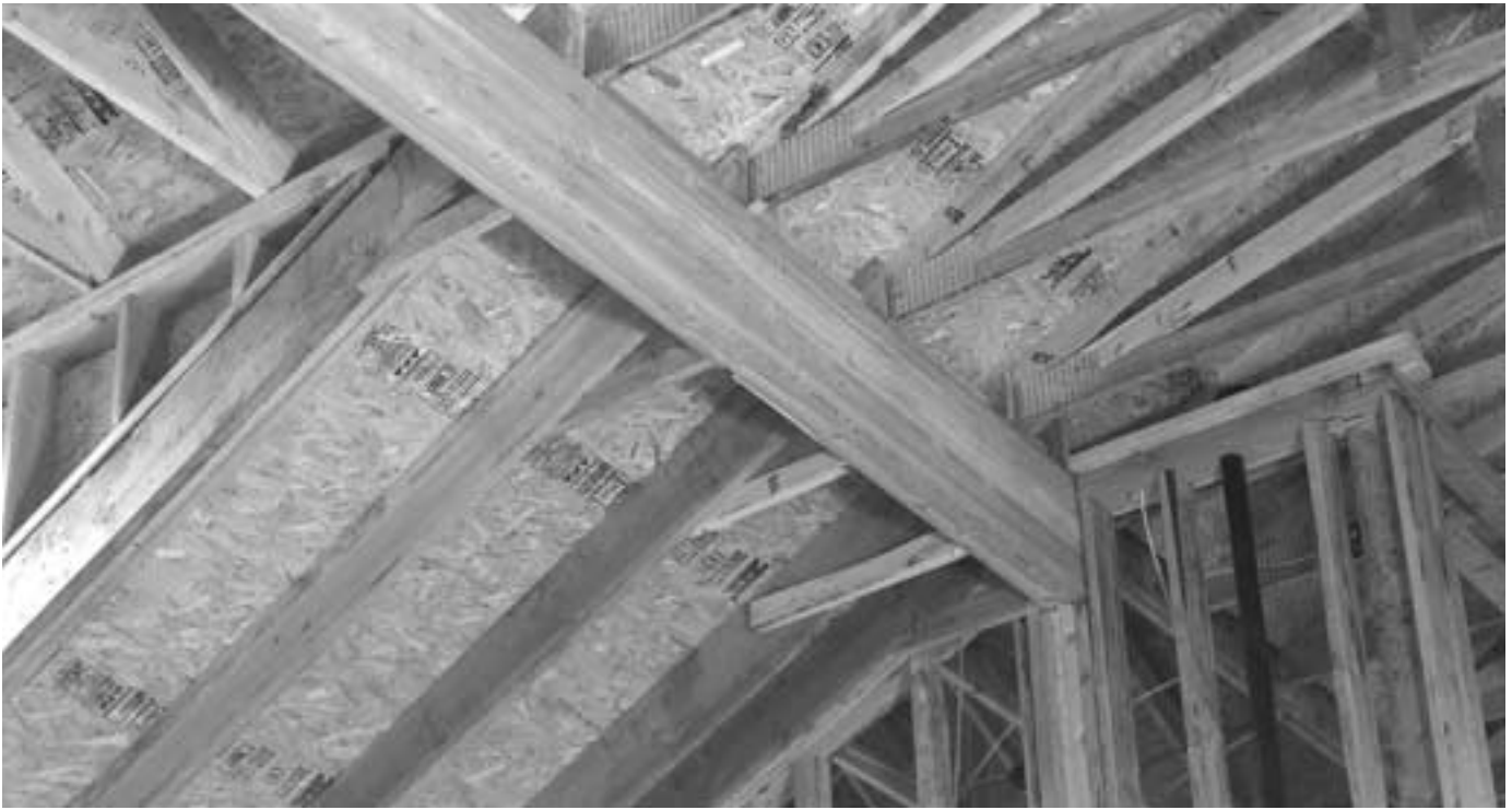
Glulam ridge beams complement the spacious, open designs common in modern residential construction. In this home, an overhead glulam beam between the dining and living rooms meets another beam in the corner to support the entire roof structure.
