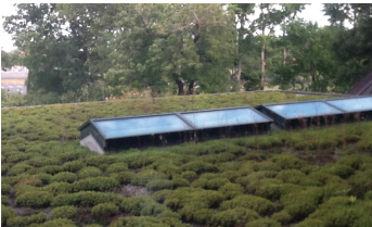
Green Roof at ICC and Leroy Meritt Center
